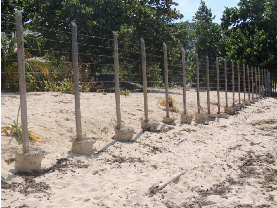
The concrete bases of these fence posts became exposed following Hurricane Sandy.
