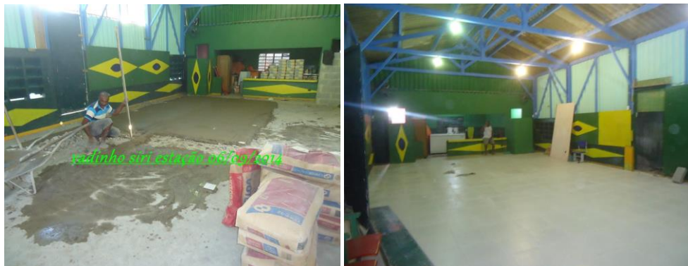
Final touch with painting. A Brazilian company, MRS Logistica, helped the Vila dos Pescadores Community Association with more construction materials to finish building the Community Centre.
